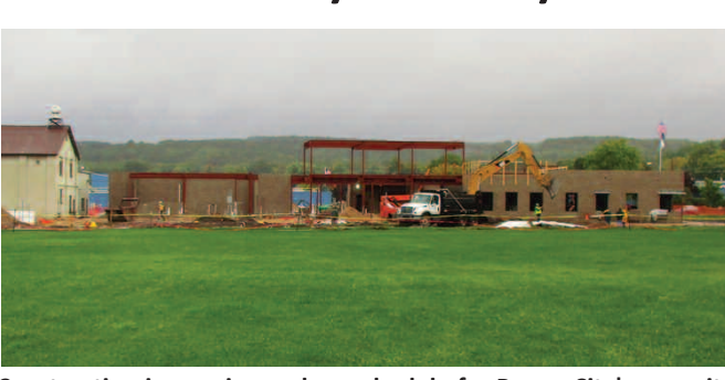
Construction is ongoing and on schedule for Boyne City's new city hall complex, which will be home to the city's administrative offices, emergency services, historical museum and MSU Extension office. The new facility at 319 Lake Street is expected to be completed by mid-summer 2017.
